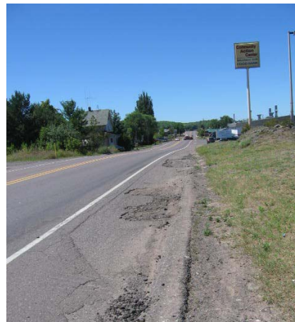
Shoulder deterioration along Sharon Ave.
